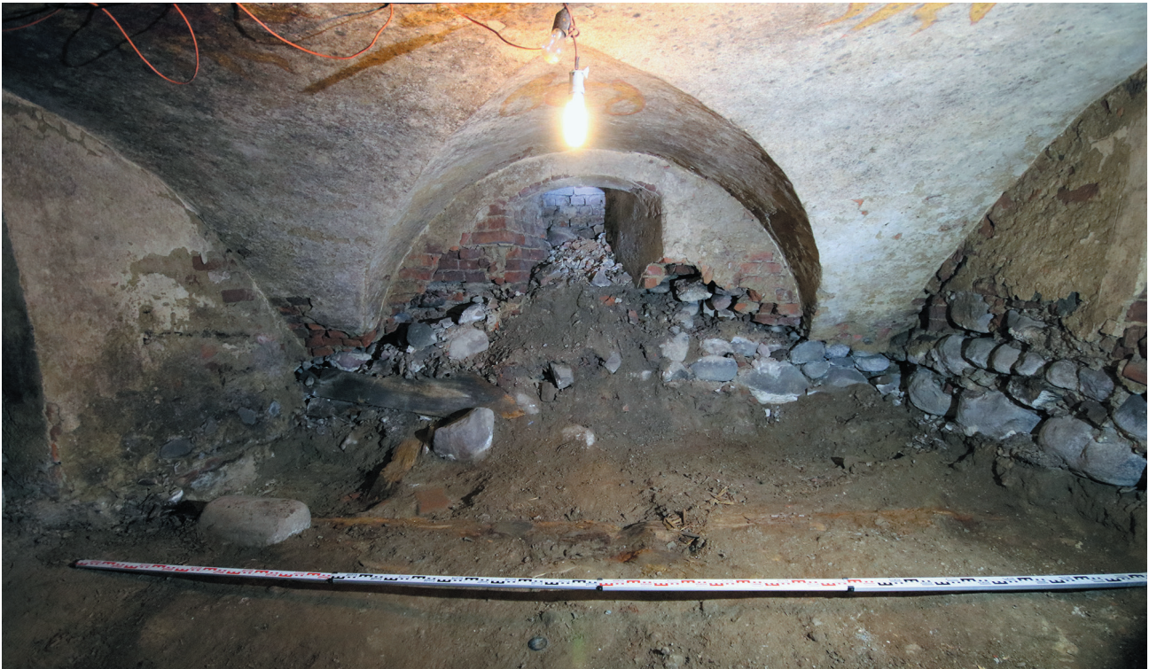
Fig. 3. The crypt's eastern wall: with a ventilation-light opening, the wall's destruction and original wooden joists visible in the crypt pugging. Photo by S. Nowak.
