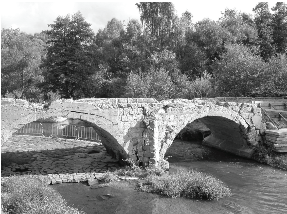
Fig. 20. View of the central part of the Zámecký (Castle) bridge in a prereconstruction state, city of Mimoň (source: VMG archive).
