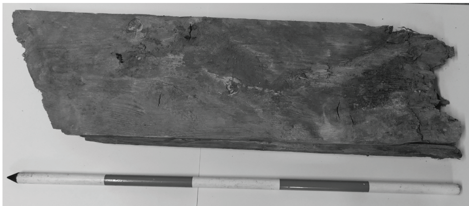
Fig. 9. A wooden plank with a groove, that was part of the formwork on the upstream side of the bridge (source: VMG archive).
