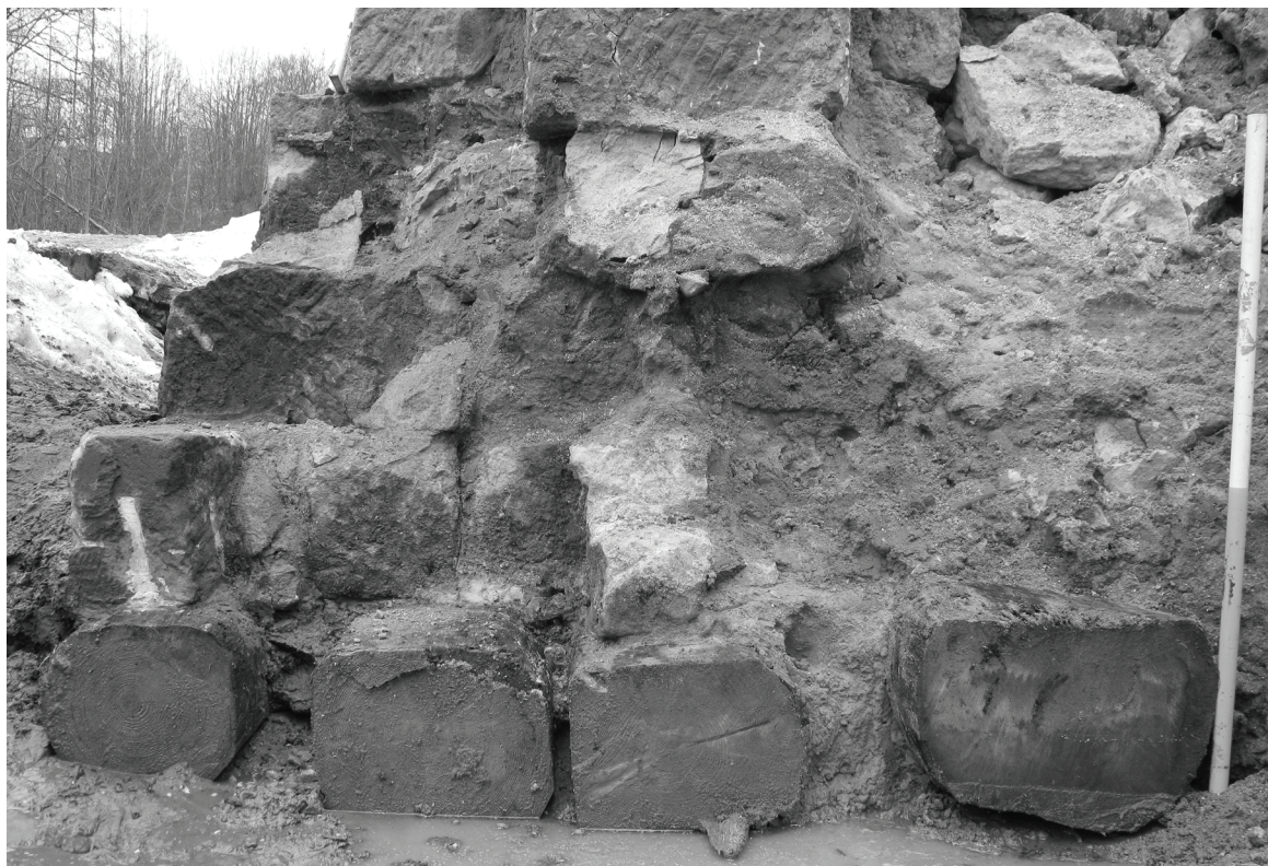
Fig. 22. The foundation of the 3 rd bridge pillar of the Zámecký (Castle) bridge (source: VMG archive).
