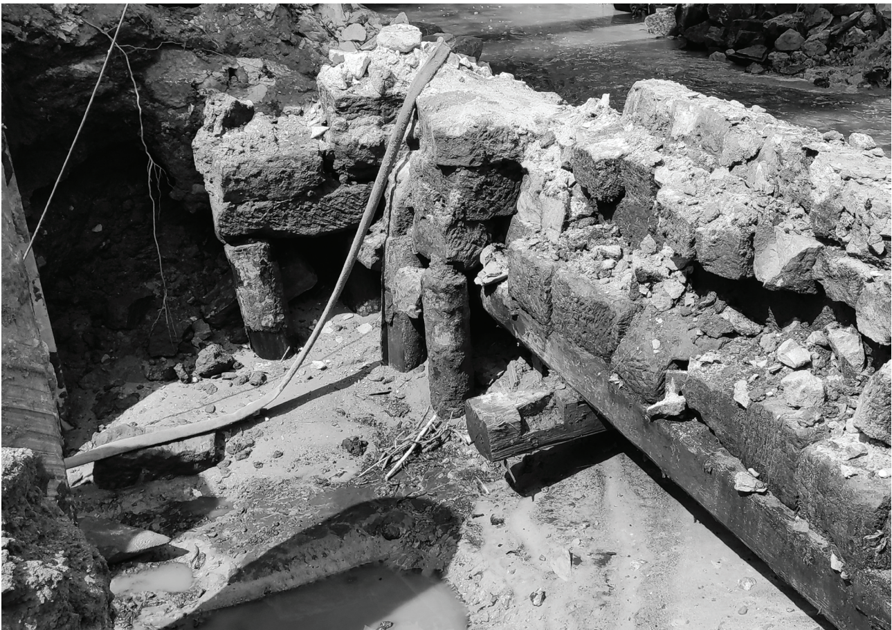
Fig. 7. View of the uncovered individual piles and grid beams under the abutment on the left bank of the stream. In the front right, a short transverse beam with mortises that were not used in the bridge construction (source: VMG archive).
