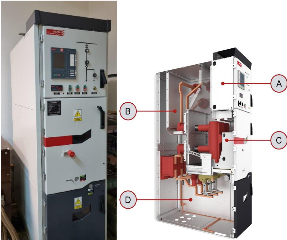
Figure 1. MV switchgear from Elektrometal Energetyka S.A.: on the left pic taken in the Laboratory of Power Apparatus and Switching Processes, on the right from (Elektrometal Energetyka S.A., 2021): A – control circuit compartment, B – busbar compartment, C – mobile module compartment, D – connection compartment.
